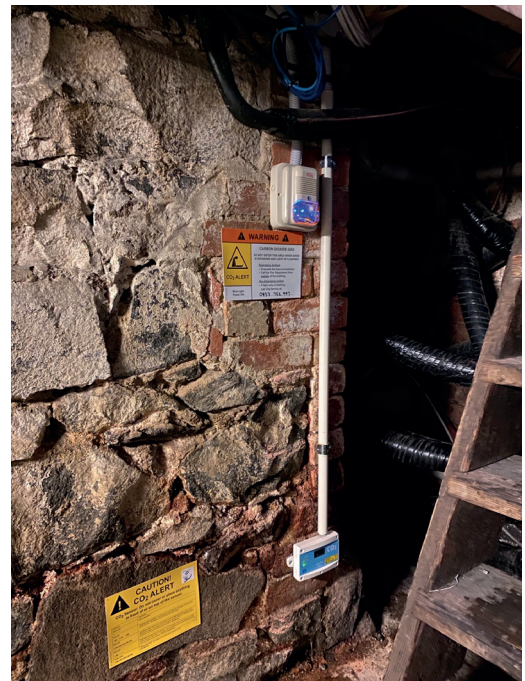
Early warning of hazardous CO2 levels before entering the cellar. Credit: Statewide Beer Systems
