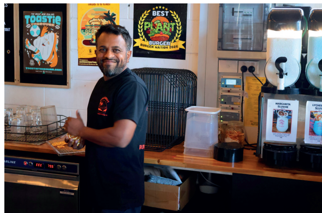
LogiCO 2 Central Unit, Power Monitor and Sniffer Bluetooth installed behind the bar as part of the CO 2 safety system
