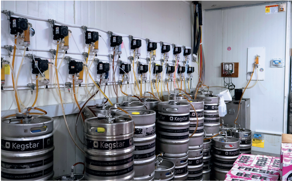
CO2 monitoring in a working beer cellar helps protect staff from dangerous CO2 levels
