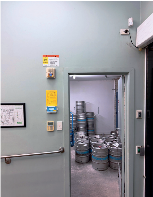
CO2 monitoring installed outside the beer cellar entrance Credit: Statewide Beer Systems
