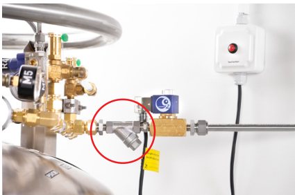
SMB and shut off valve installed with filter
